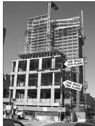
The Raw Space: Here's what the space looked like as of late September, 2006.
