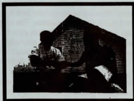
Jeff Williams and Alex Bess up on the roof on Block Island
